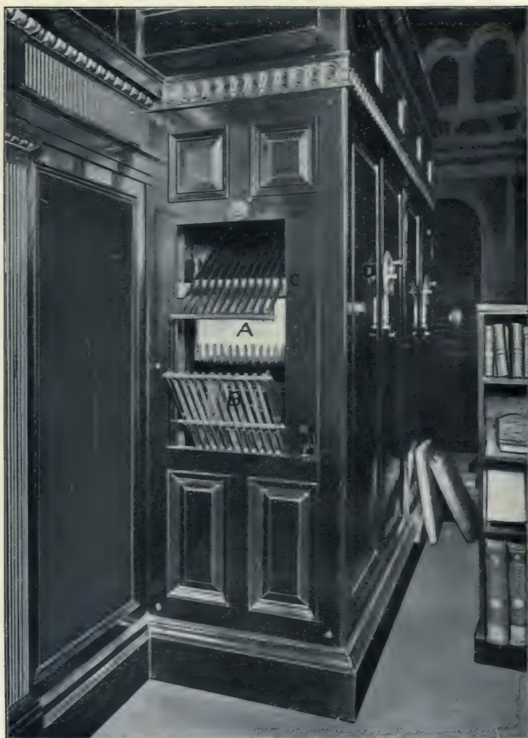
BOOK CARRIER TO SOUTH STACK (NO. 4), READING ROOM TERMINAL. MAIN FLOOR, ROOM U3 OF PLAN.
